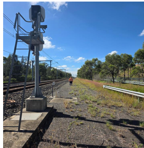
Image 5: Inner HS Location to protection placed at 45.055 KM
