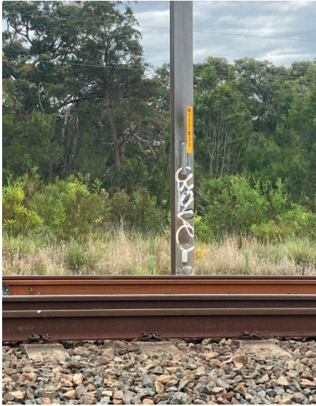
Image 1: Sensor installation reference location
