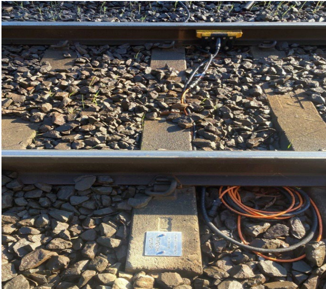
Image 1: Transmitter and sensor installation location
