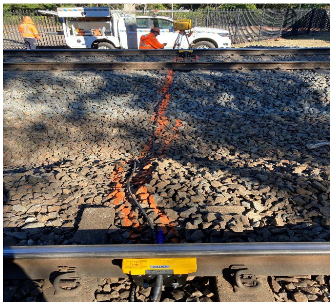
Image 1: Transmitter and sensor installation location
