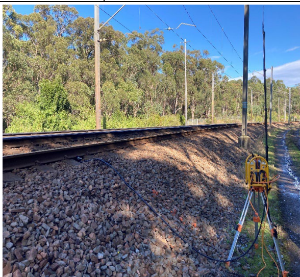
Image 1: Transmitter and sensor installation location
