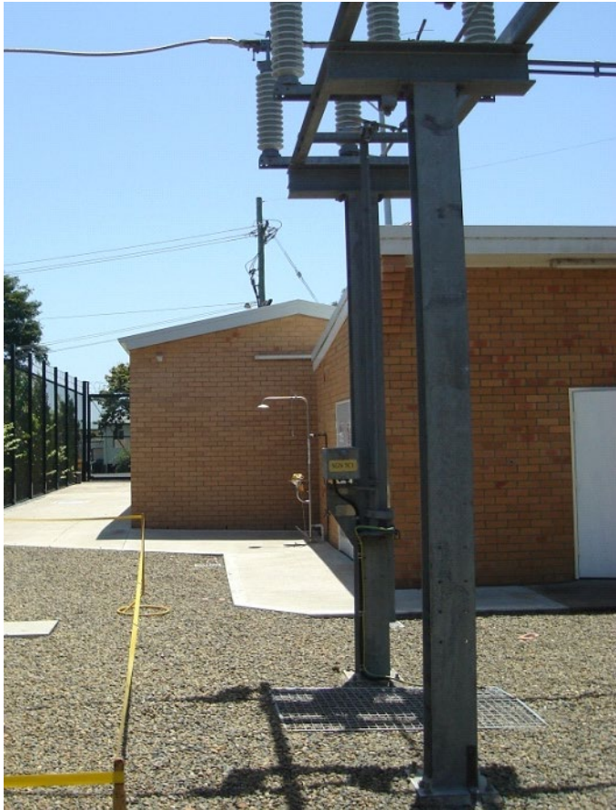
Figure 5: Tape is supported by stands, NOT high voltage structures
